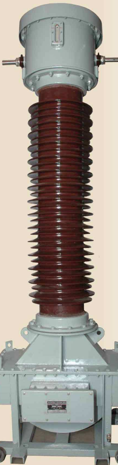
132KV DEAD TANK CT
