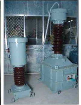
High Voltage Testing
